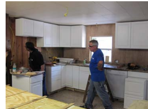
Brand new cabinets, counters, and appliances are installed to finish Herman's kitchen.
